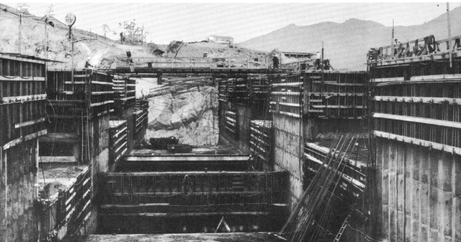
High and low blocks in high and low rows—Note use of cantilever type forms
