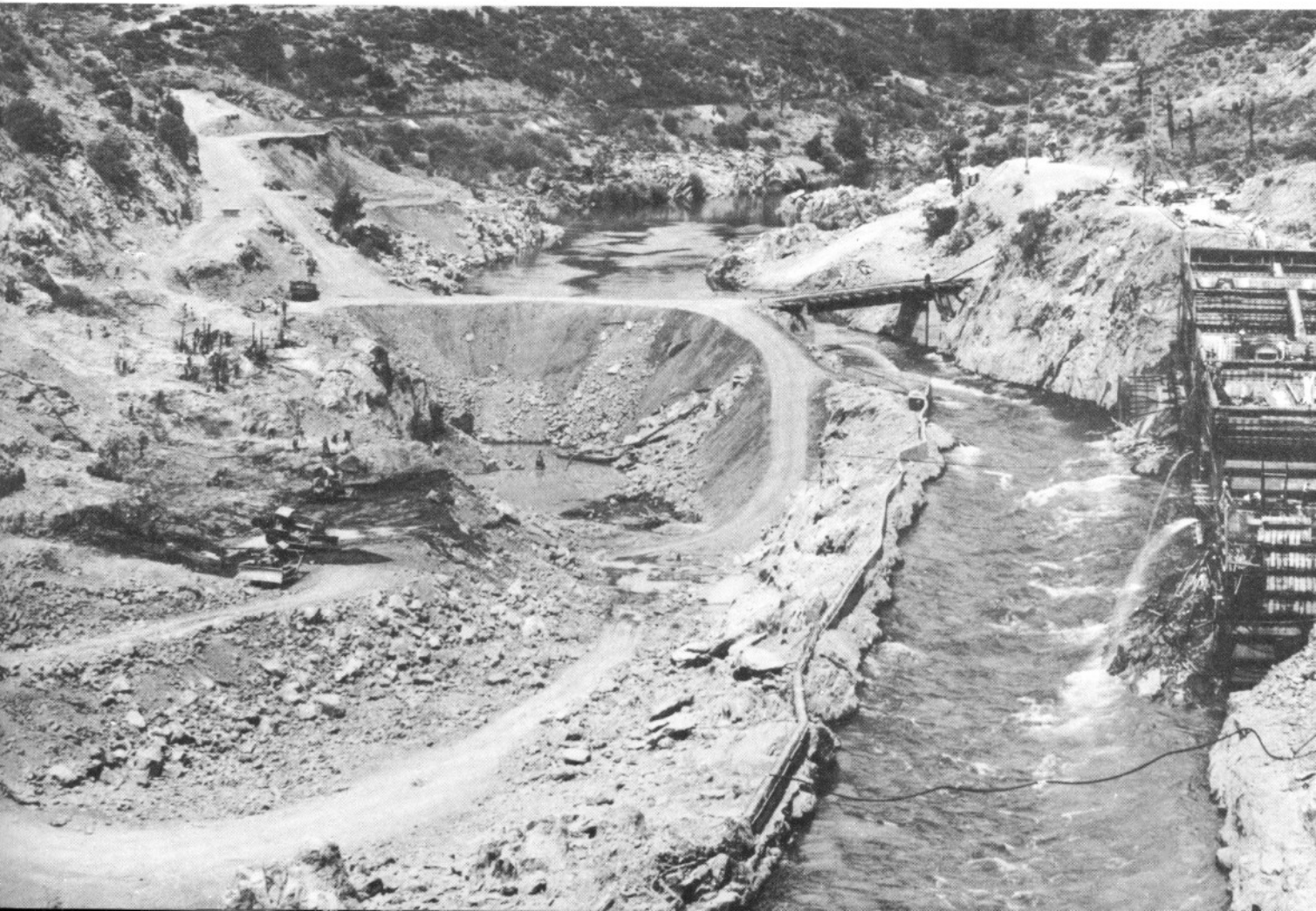
River diverted through channel on east side while excavating river bed, August, 1940
