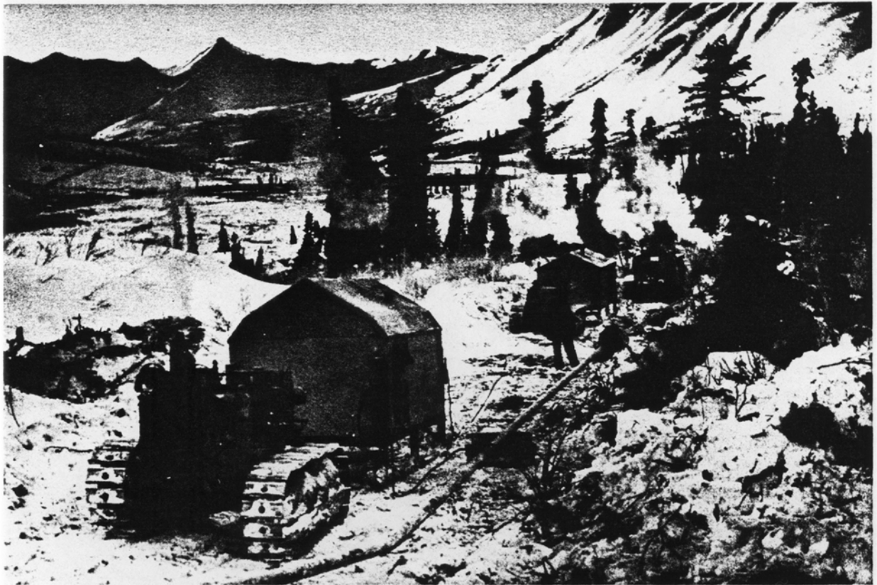
Welding of the Canol Pipe Line was continued even at temperatures of 60° below zero.
