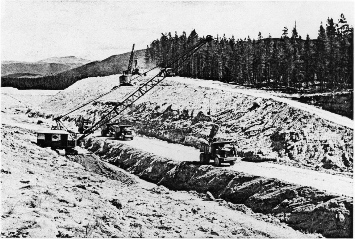
Wet materials including quicksand was removed in digging the Granby Pump Canal high in the Rocky Mountains.
