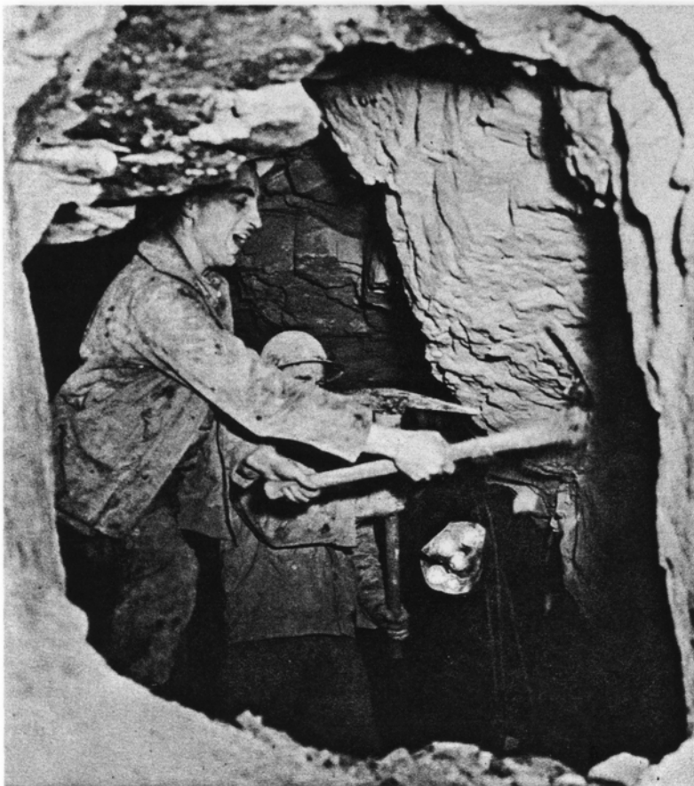
Holing through on the San Diego Aqueduct for the United States Navy.
